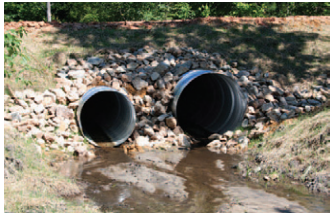
Figure 12: Following Virginia's Best Management Practices helps ensure the protection of water quality. These culverts are part of a well-planned stream crossing.
