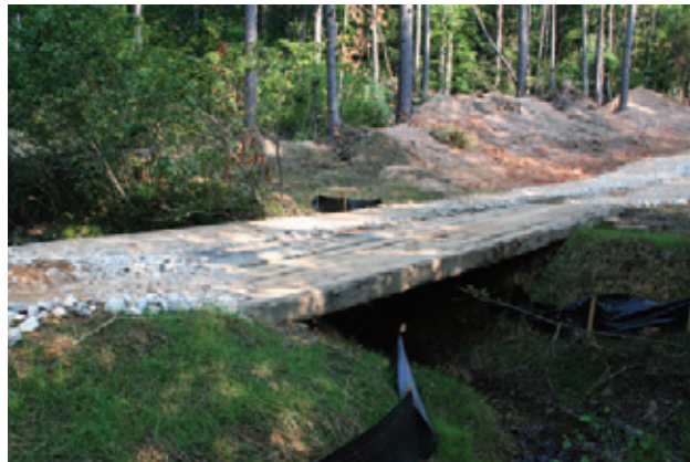
Figure 6: Proper stream crossings are an important part of protecting water quality. Notice that, in addition to the bridge, the stream banks have been seeded to reduce erosion.
